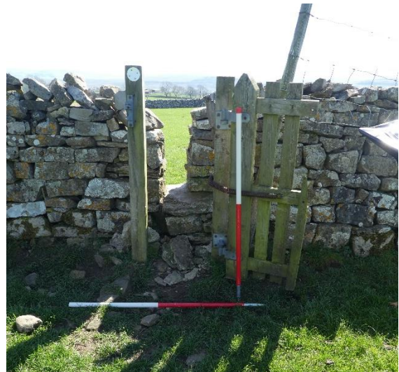
Figure 23 Squeeze stile (A073) that requires a more considerable step up.
