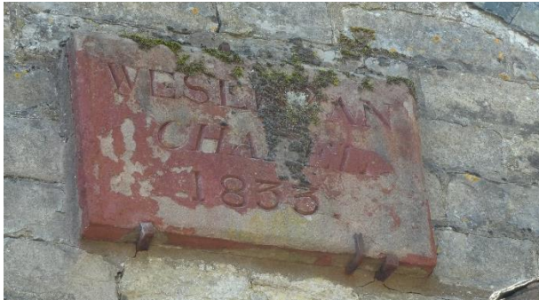
Figure 10 Date stone on the Wesleyan Chapel (G071a) - the inscription is becoming obscured by lichen and weathering.
