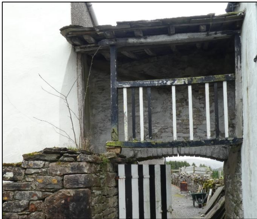
Figure 11: Feature B24 a former gallery located over a public right of way.
