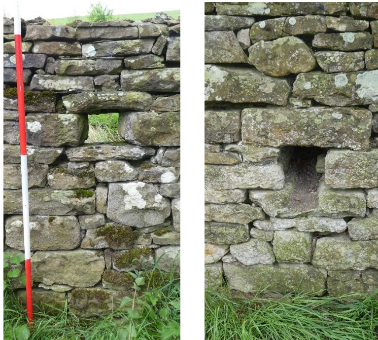
Figure 13: Right – Unknown hole in a dry stone wall (F016) possibly associated with the deer park. Left – Unknown hole in dry stone wall (F017) with shaped/bevelled base.
