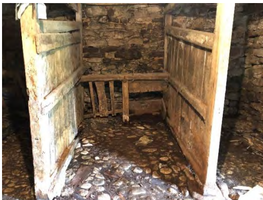
Figure 46 Evidence of larger stall dividers and fallen hayrack.
