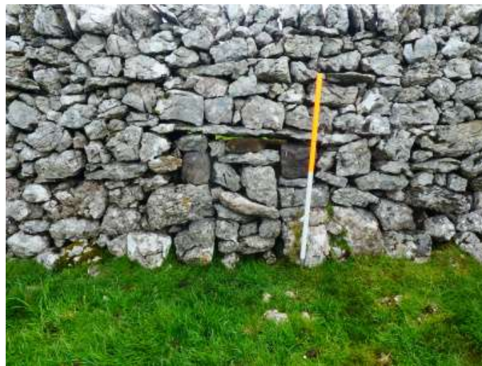
Fig. 47 Wall no. 13 with a blocked sheep creep, looking east (1m scale)
