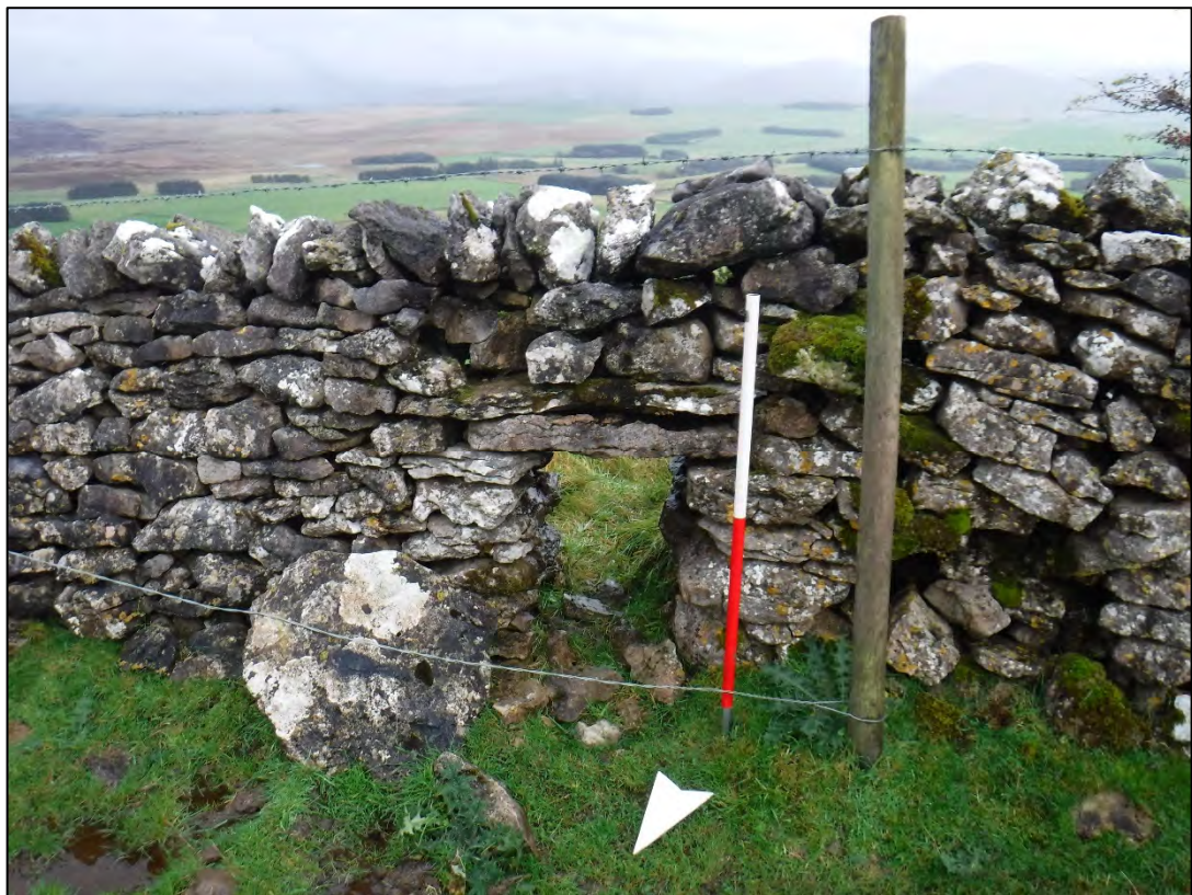
Plate 42: hogg hole C73 is still in use. The stone slab has been set aside to let the yearlings through.
