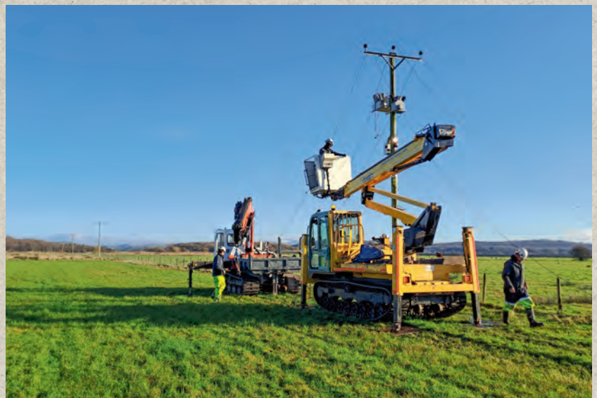
Lines coming down at Meathop © SP Energy North West
